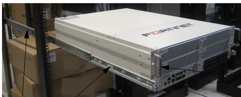
Figure 11: FortiGate unit halfway on rack showing release tabs.
