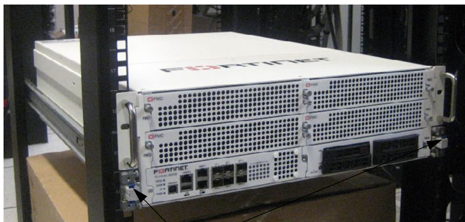
Figure 12: FortiGate unit on rack.
